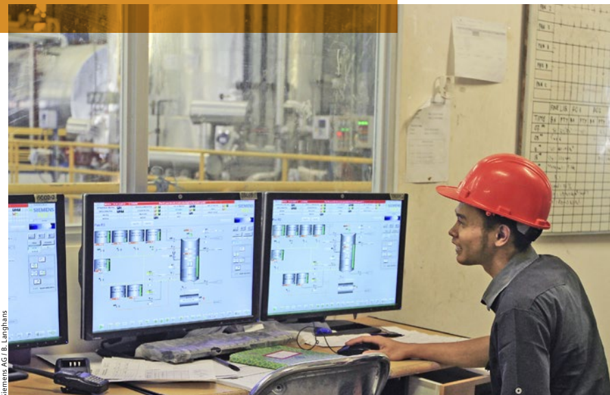
The new control room of the sugar plant
