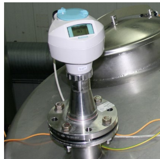
Sitrans LR250 HEA mounted on a cream tank
