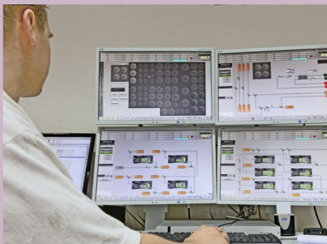
The tank farm manager uses intelligently designed routines to support the user in the process of moving items in and out of storage. The application is based on Simatic Route Control
